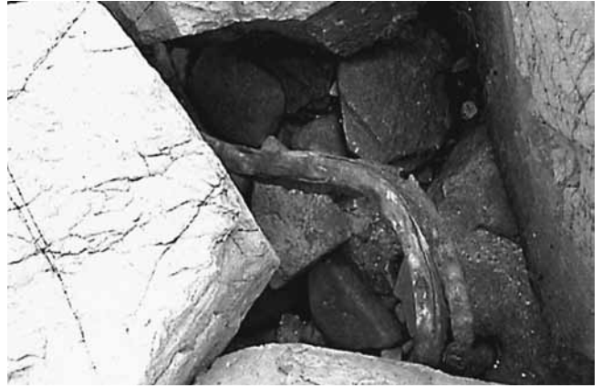
Figure 21. Steel rail lines from slipway twisted by the weight of the rock infill c.1999.
