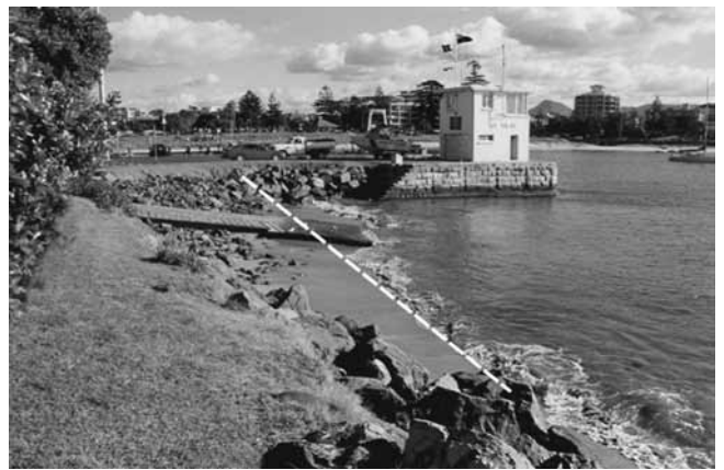
Figure 22. Location of the seawall before the storm damage (white dotted line), 2004, (looking south-west).
