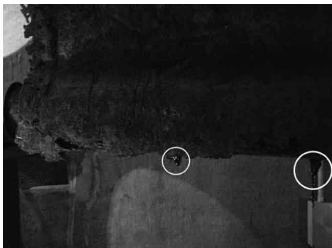
Figure 14. Starboard view of Defender's exterior stern bilge; highlighted areas show unidentified resinous substance that emerged from the hull during a warm weather event and later re-solidified. The vessel's screw aperture is at far left of image (Photograph by the author).
