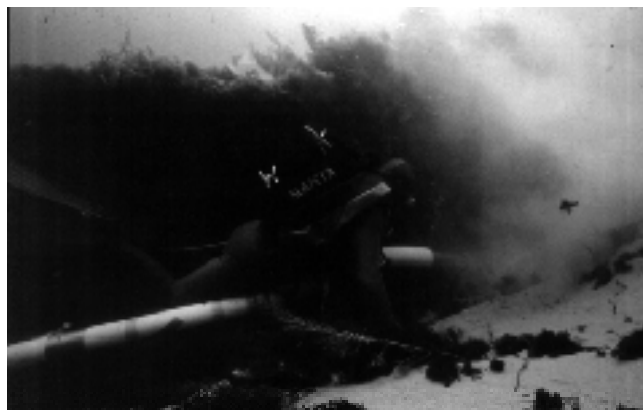
Figure 2. Attempt to fill scour holes by underwater sediment dredging. Note the large amount of suspended sediment.
