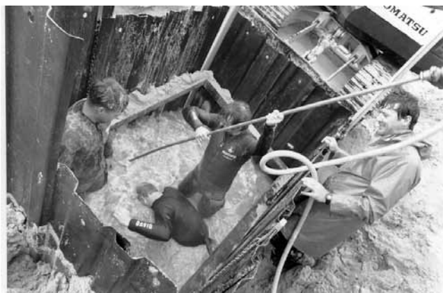
Figure 11. The iron artefact could not be uncovered and could only be reached by loosening the sand with the air probe and reaching down by hand. (Photo: S. Humphries)
