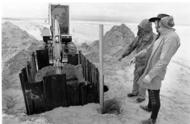
Figure 10. Extraction of sand caused subsidence in the area surrounding the caisson. (Photo: S. Humphries)
