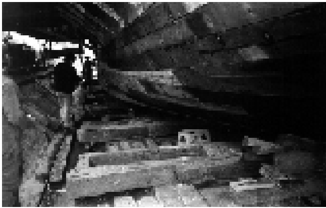
Figure 2. The PS Marion sitting in the dry dock showing the new planking added to the vessel, and the original planking and trestles of the dock. (Courtesy: Mannum Dock Museum)
