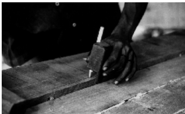
Figure 7. Carpenter using a mortise gauge to indicate the wood to be removed.
